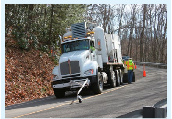
DBI's (IRM) Road Management Unit utilizes the industry's only fully automated HFST application vehicles, which can apply HFST continuously at full lane width.
