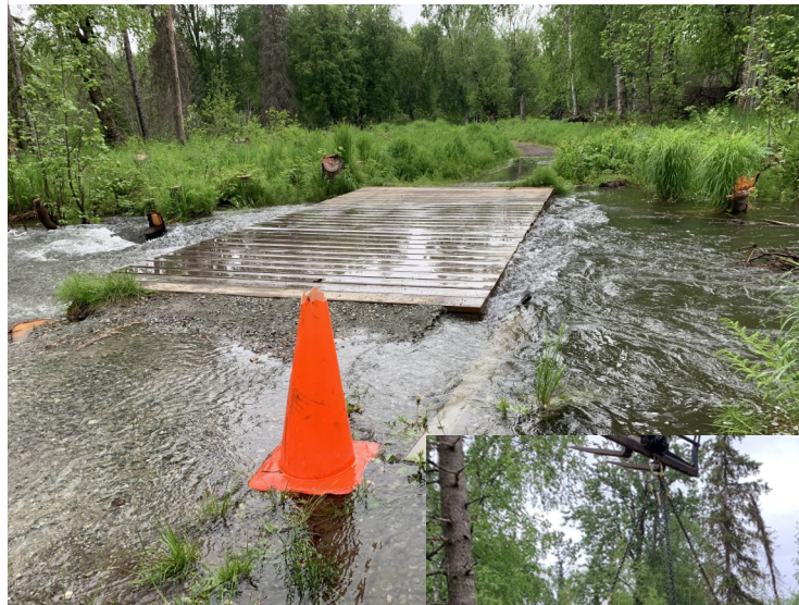
Left: High water near the existing South Fork Side Channel Bridge
