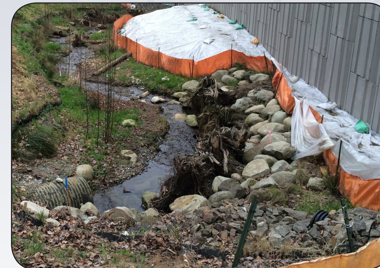
Roughened toe near SR 520 in King County, Washington, 2014.
