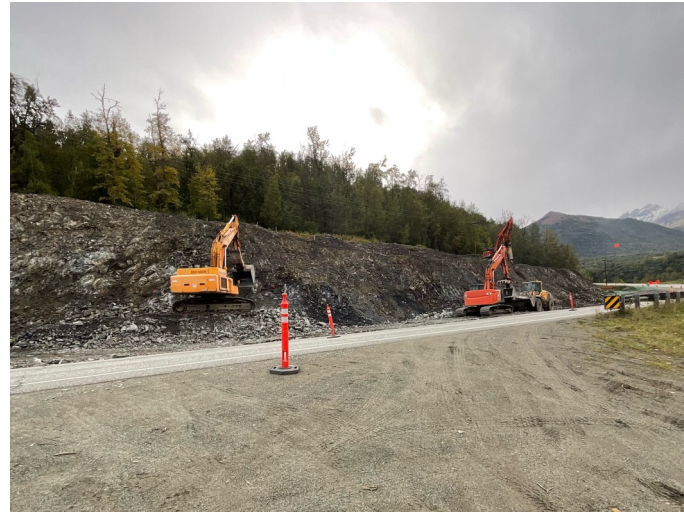
All Project Images Source: FHWA
