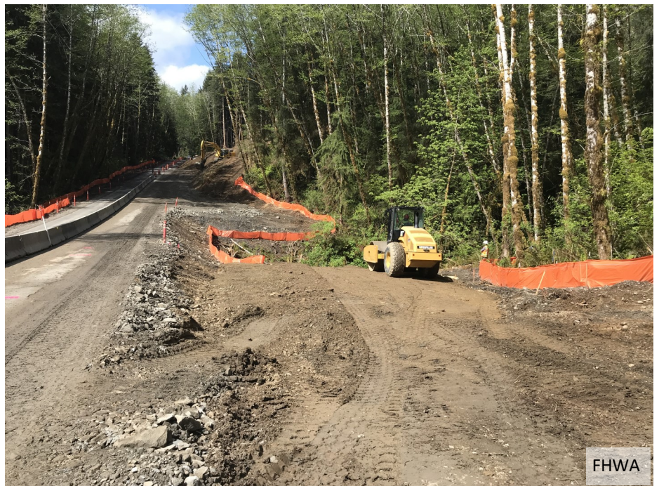
Placement and compaction of backfill material at the location of the West approach and abutment of the future bridge
