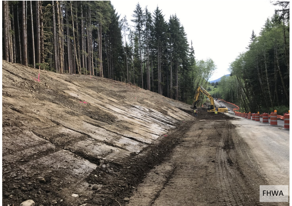
Excavation and shaping of the slope at the hillside on the northwest side of Canyon Creek.
