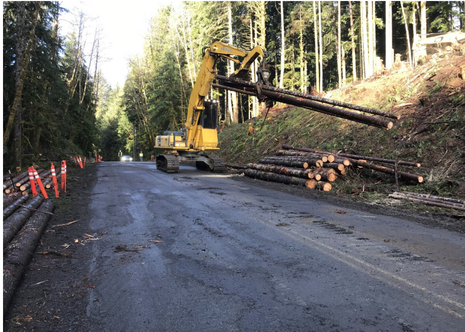
Clearing of trees at Canyon Creek. Many of the larger logs will be reused as part of the Engineered Log Jams
