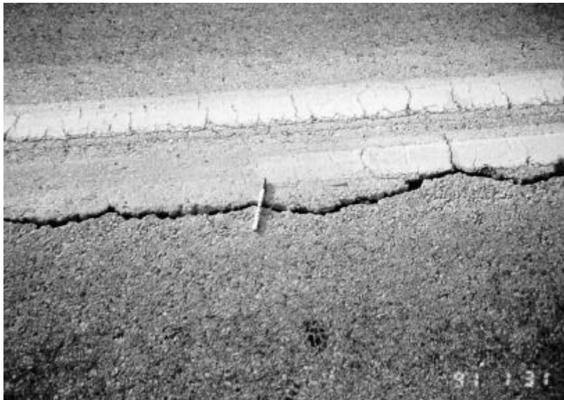
Figure 5. Pavement candidate for longitudinal crack filling.
