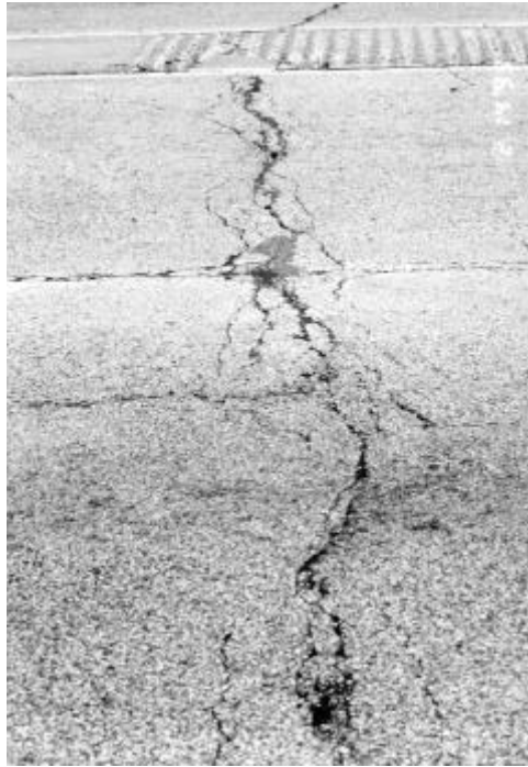
Figure 3. Pavement candidate for crack repair.
