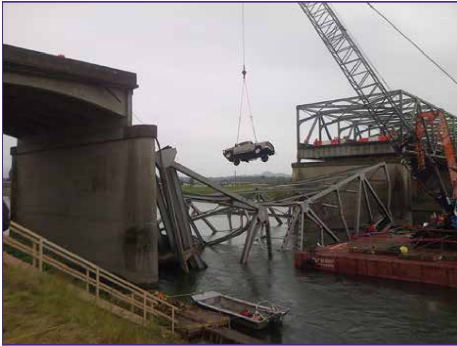
Here, a crane hoists a pickup truck from the river. The truck plunged into the water when span 8 of the bridge collapsed.
