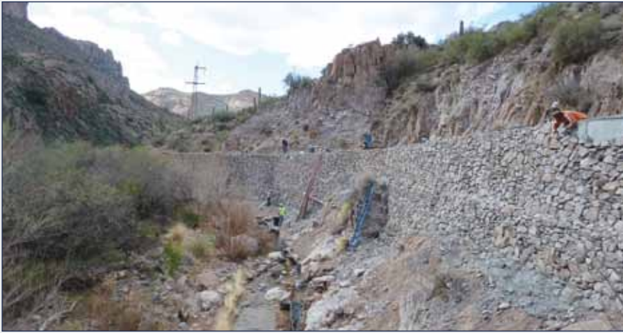
Maintenance crews are repairing a historic retaining wall along a segment of State Route 88, also known as the Apache Trail, in Arizona.
