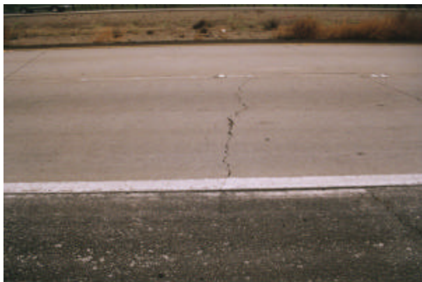
Figure 3.1.10 Medium severity transverse crack at 06-CS1, Tracy Test Road (control section).
