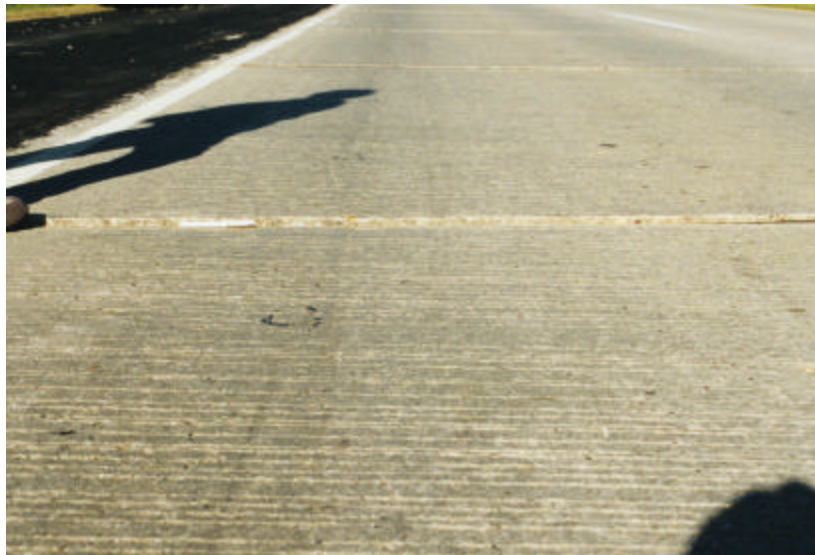
Figure 4.2.1 Faulted transverse joint in test section 55-3008.
