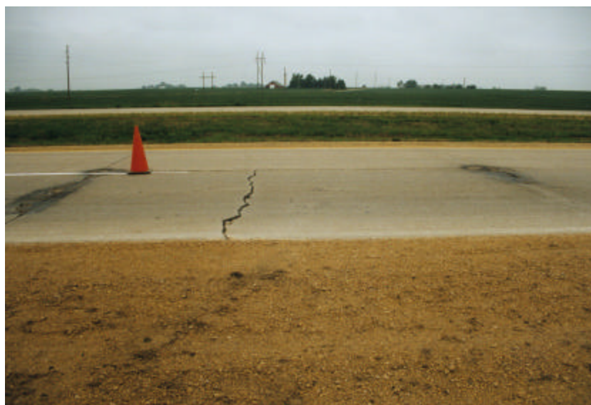
Figure 4.3.5 Transverse cracking closer to the leave joint for the Iowa section 19-3006.
