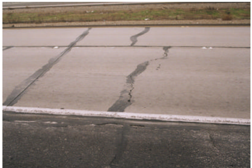
Figure 4.2.5 Depressed shoulder in test section 06-CS3 from pumping of fines. Transverse cracking in outer and inner lane.
