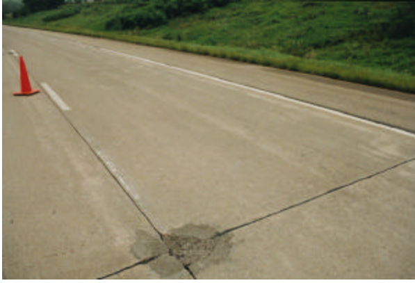
Figure 3.1.23 Corner break and repair at 27-4054.
