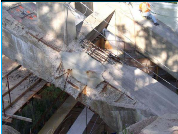
Figure 1. Freeze-thaw deterioration at Castlewood Canyon. 1
