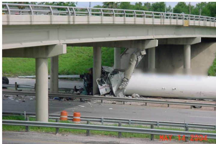
Figure 3. Photo. Truck impact on piers of Tancahua Street Bridge over IH-37, Corpus Christi, Texas on May 14, 2004.
