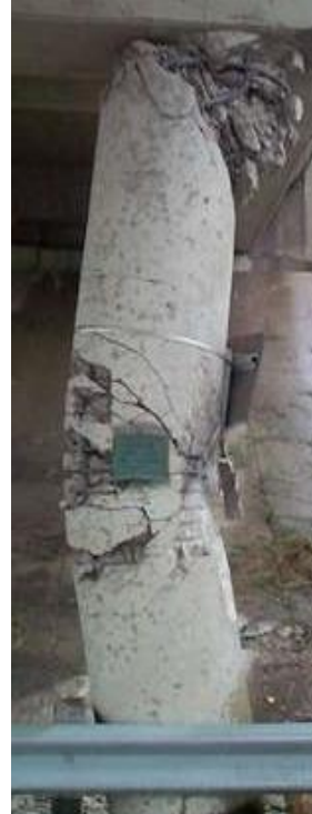
(b) Minnesota I90 bridge accident (2003).
