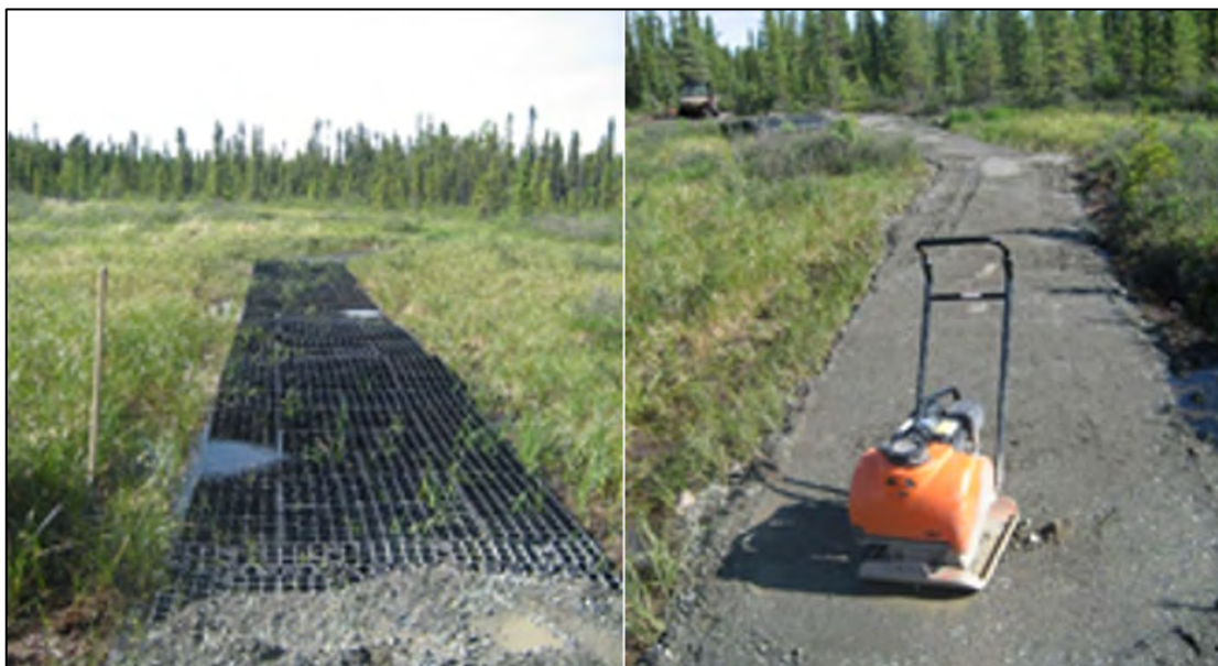
Figure 8: GeoBlock infilled with gravel used in trail construction for the Copper Lake Trail during construction (left) and after (right) (Source: NPS)
