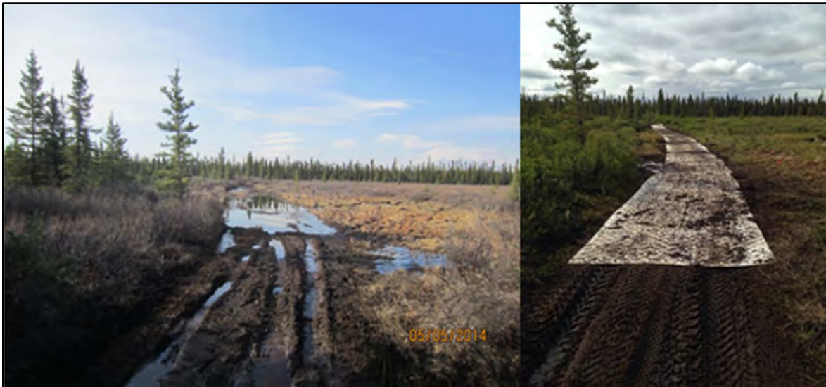
Figure 6: DuraDeck used in trail construction for the Copper Lake Trail before (left) and after (right). Source: NPS
