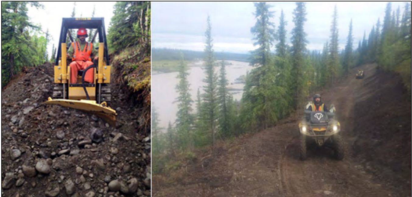
Figure 9: Bench cut used in trail construction for the Copper Lake Trail during construction (left) and after (right) (Source: NPS)
