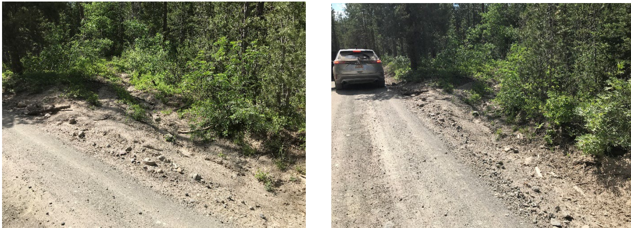
Figure 20: Evidence of water runoff chutes at MP 17.0 during July 2022 Site Visit
