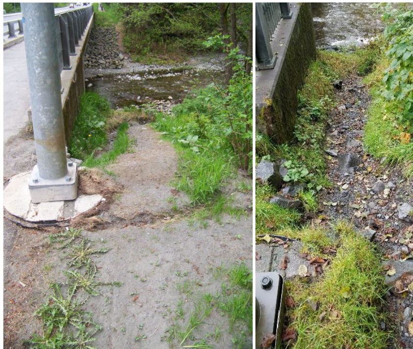
Figure 8 - (L) Trail connection in 2014. Water started to wear channels into the soil. Figure 9 - (R) Trail connection in 2018. Trail surface has continued to deteriorate and large rocks are starting to show through. The surface is very loose with uneven footing.
