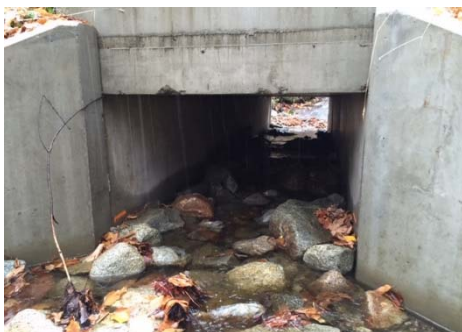
Rehabilitated culvert at Silvio O. Conte NWFR – Nulhegan Basin. Photo by FWS
