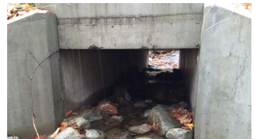
Rehabilitated culvert at Silvio O. Conte – Nulhegan Basin Division provides stormwater management and aquatic organism passage.
