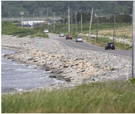
Road rebuilt after Hurricane Sandy at Sachuest Point NWR. Photo by FWS
