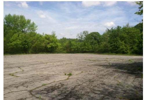
Deteriorating parking lot at Ohio River Islands NWR considered for partial decommissioning. Photo by FWS
