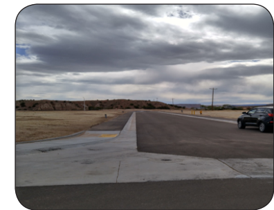
Pueblo of Jemez – Pueblo Place Subdivision, New Mexico Construction of roadways, sidewalks and installation of lighting
