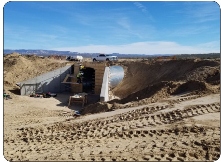
Pueblo of Zia – Cabezon Road, New Mexico Grading and Drainage Improvements, installation of cattleguard underpass, guardrail, realignment of roadway, road grading and culvert drainage installation
