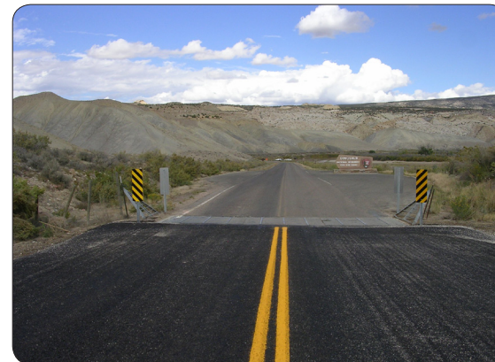
State Route 149, Utah State Route 149, a rural collector leading from US 40 to the western entrance of Dinosaur National Monument, is the main access to Dinosaur National Monument from Utah. This FLAP project widened the existing facility to 12-foot lanes with 4-foot shoulders and included 17 culvert replacements and a bridge replacement.
