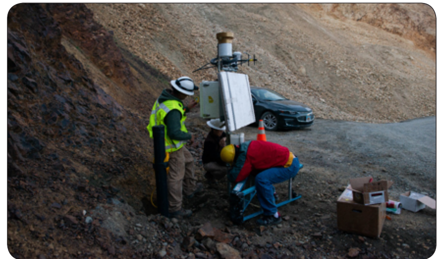
Turner-Fairbank Highway Research Center and WFL geotechnical personnel worked together to install the communication base station for the drill hole monitoring equipment, rain gauge, and air temperature equipment just outside the western limits of the landslide.
