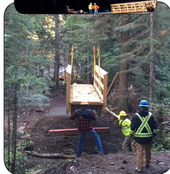
Workers guide the bridge into position, coordinating with the helicopter pilot for placement.
