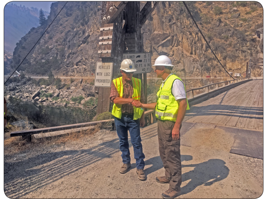
Tim (right) onsite at the Manning Crevice Bridge Replacement project presents Western Federal Lands Project Engineer, with a Federal Lands commemorative coin, for a job well done! — Salmon River Road, Idaho
