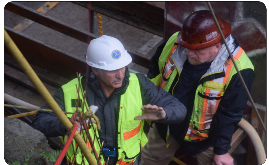
FLH Geotechnical Engineer consults with on-site staff on the construction of the new George E. Tryon Bridge, South Fork Smith River Road, California
