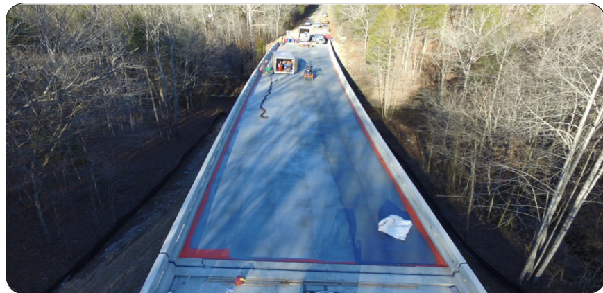
Top Left: Application of prime coat; Right: Application of polymer membrane Bottom: Application of top coat
