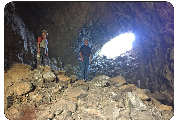
Scoping Trip inspecting another railroad tunnel slated for an upcoming project, further along the Spruce Railroad Trail.
