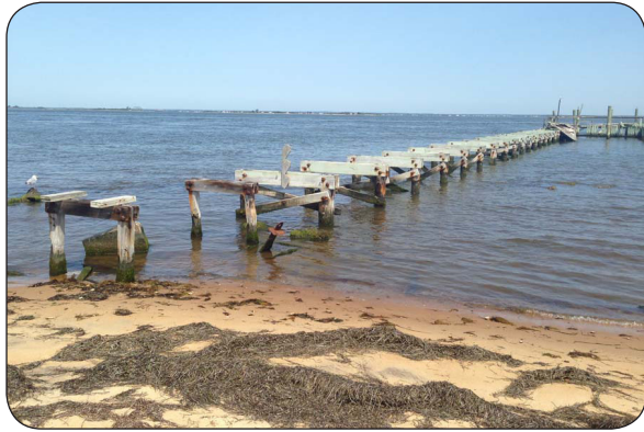
Lighthouse dock after Hurricane Sandy
