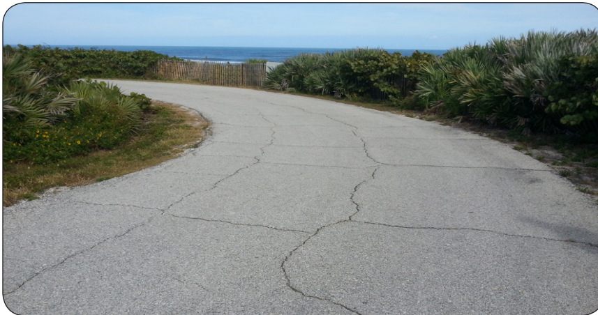
View of a stretch of roadway condition showing visible cracks, a condition suitable for pavement preservation treatment as a low cost alternative to extend the life of the pavement at Canaveral National Seashore, Florida
