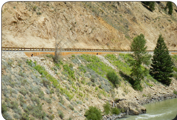
View of the stained shotcrete facing above the roadway
