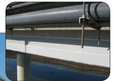
Close-up of beams after repairs were completed and the finish coat was applied
