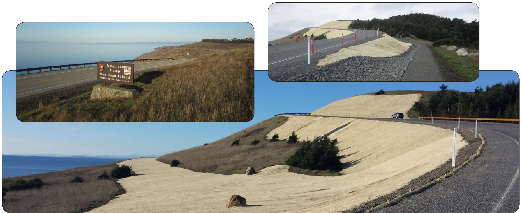
Views of the realignment, the original road location will soon be filled in with native vegetation leaving the scar barely visible
