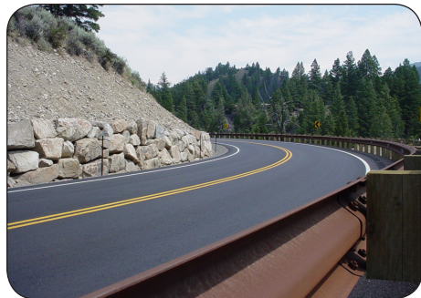
Stained stone retaining walls and guardrails
