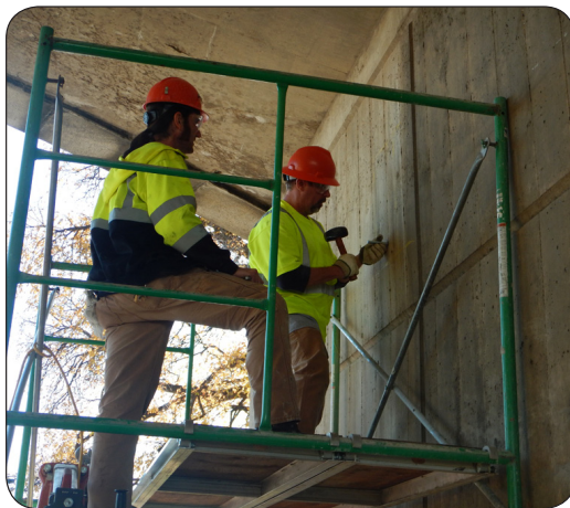
Bridge Inspection staff drilling concrete test core samples from bridge abutment for in-depth investigation at Pentagon Reservation, Arlington, Virginia
