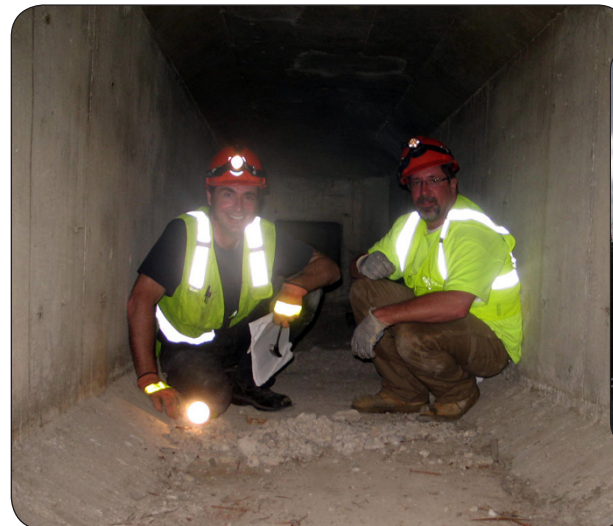
Bridge Inspection staff conducting routine inspection of concrete box girder at Smithsonian National Zoo, Washington, DC
