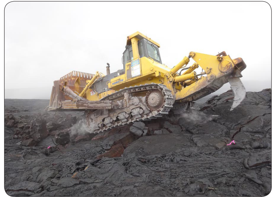
Bulldozer as it begins to cut through the lava for the new roadway alignment
