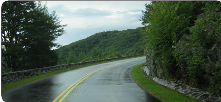
Though not as prevalent in other federal land units, stone paved waterways are common drainage features along the Parkway
