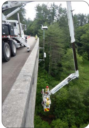
BIP "Snooper" vehicle in use, wind meter mounted on bridge is monitored remotely, Blue Ridge Parkway, VA
