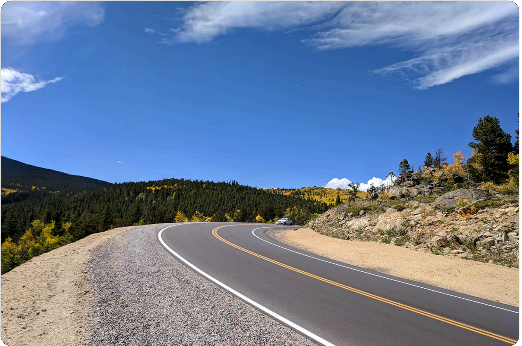
Brainard Lake Road Project improvements included widening to accommodate cyclists, drainage, sight distance and upgraded signage and striping. Brainard Lake Recreation Area, Arapahoe and Roosevelt National Forests, Colorado
